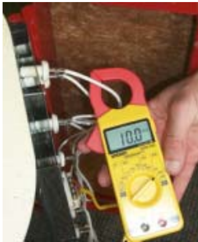
Testing Amperage at Feeder Wires
